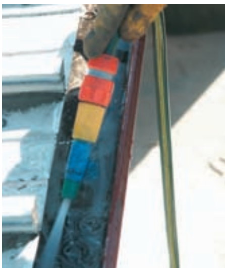
4) Rinse the gutter with water to soften and break up the dirt.
