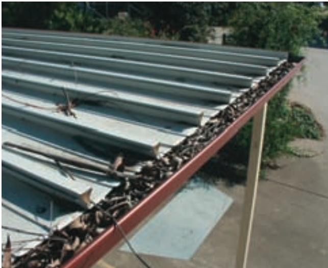
1) A typical suburban roof with leaf litter and dirt prior to cleaning.
