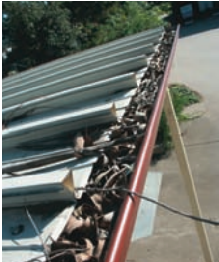
1) A typical suburban gutter clogged with leaf litter prior to cleaning.
