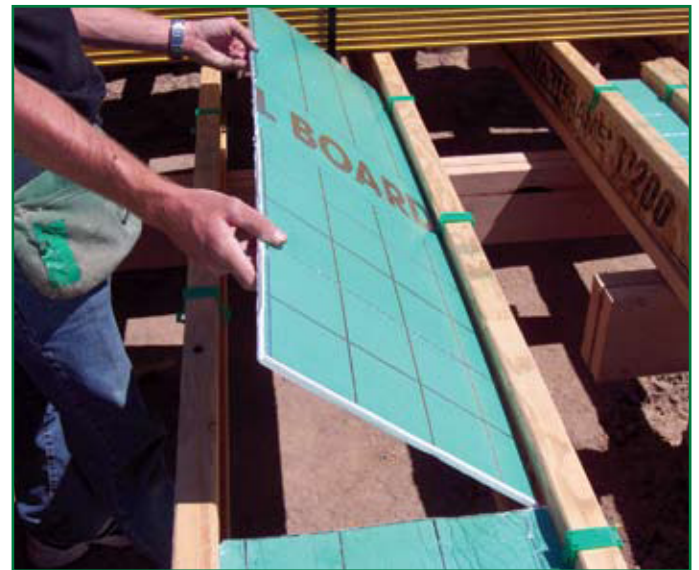
FOILBOARD® INSULATION PANEL is being used in conjunction with the FOILBOARD® FLOOR SADDLE during the construction process. Note the ease of application.
